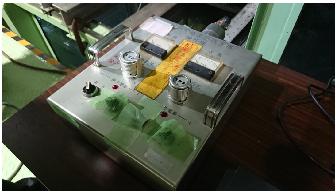
Fig. 4-2 The Circulating Water Channel control panel
