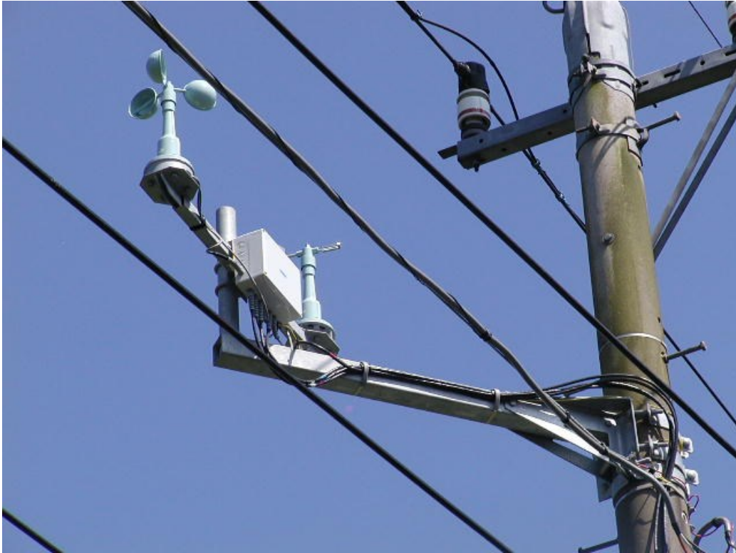
Photo 3.3 Anemometer and wind vane
