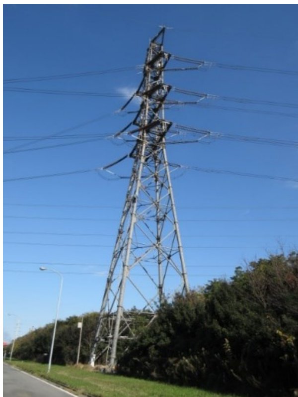
Photo 1.1 Overhead transmission line
