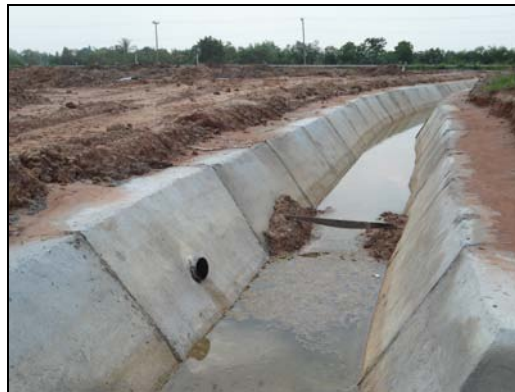
Figure 3.24 Sub-surface drainage system at Khon Kaen province, Thailand
